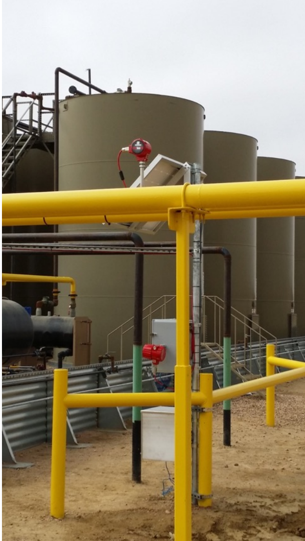
Figure 3. Flowmeters, like the QuadraTherm 640i units shown here, measure the flow of gases at a flaring unit
